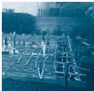
Radiant Floor Heating
